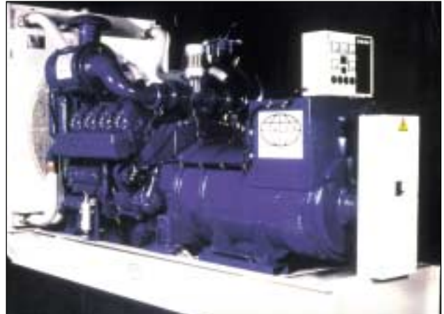
Diesel generator sets. Couplings fitted between diesel engine and alternator.
