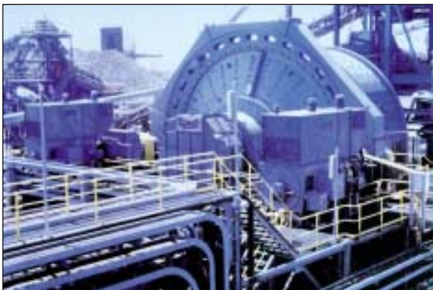
Grinding mills. Couplings fitted between electric motors, gearbox and mill.
