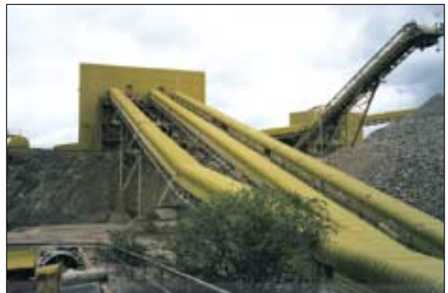
Conveyor drives. Couplings fitted on belt conveyor drives.
