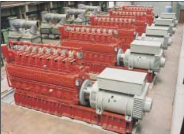
Bio-gas generator sets. Coupling fitted between gas engine and alternator.
