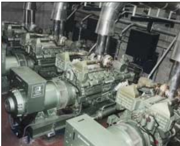
CHP plants. Couplings fitted between diesel engines and alternators.
