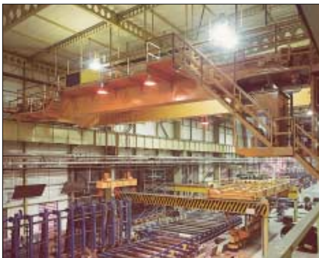
Steel mills. Couplings fitted on 35 tonne overhead crane, and on table roller drives.
