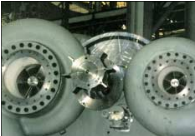
Compressor drives. Coupling mounted between electric motor and compressor input shaft.
